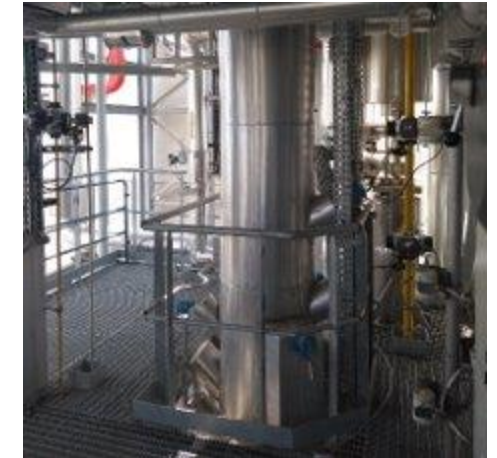
Methanation reactor installed at the GAYA platform
